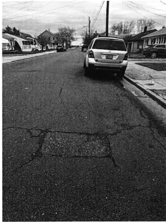
Photo 5 – Patched area exhibits differential settlement and cracking / separation along the edges of the patched area.
