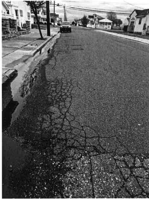
Photo 7- Poor drainage along the shoulder has contributed to premature deterioration of the asphalt surface.
