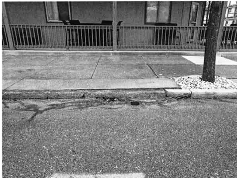
Photo 8 – Deteriorated asphalt in an area exhibiting poor drainage
