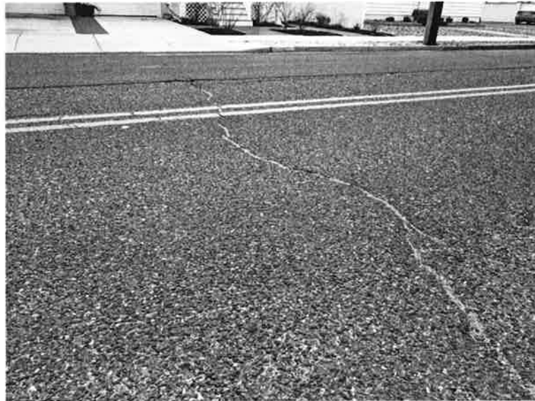
Photo 1 – Typical transverse crack
