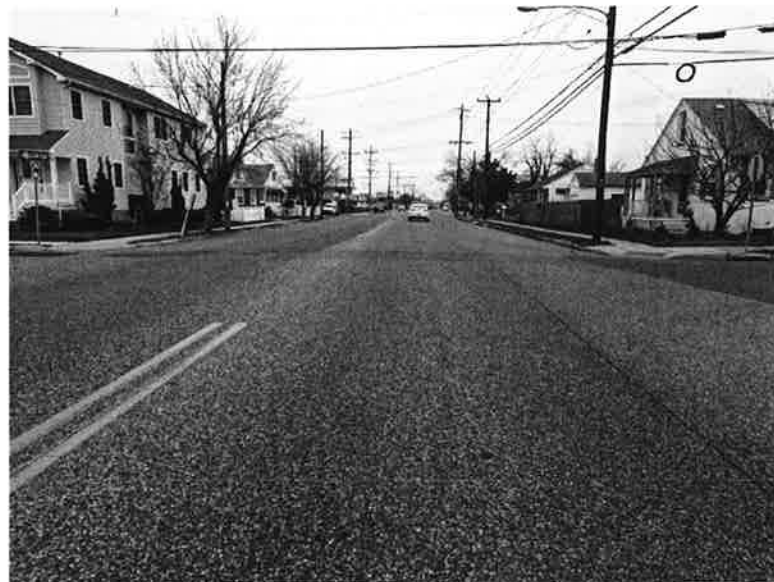
Photo 2 – Typical longitudinal crack
